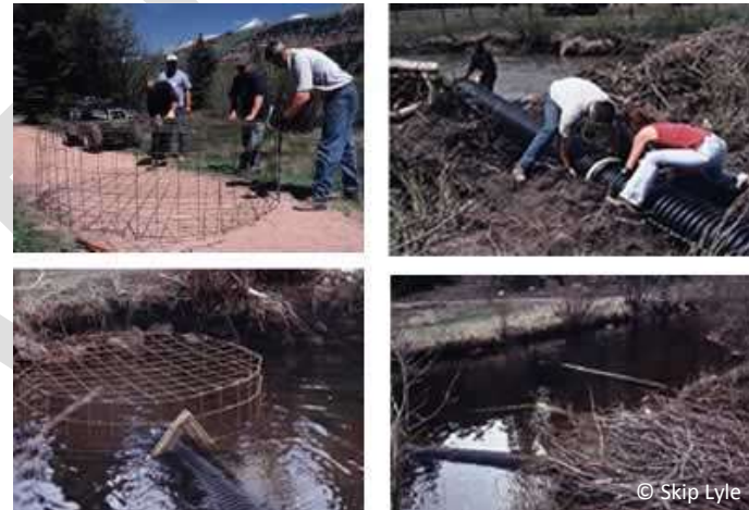
Inserting a flow regulator into a dam to control the pond water level.
